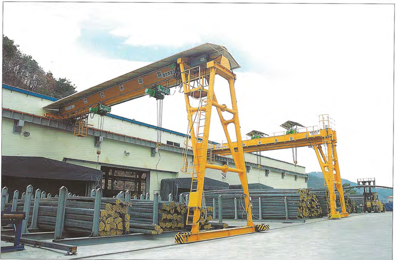
1st Rebar Processing Factory
